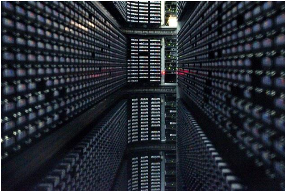
Interior of a digital tape library
